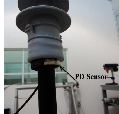
Fig. 7 Position of the sensor in the terminal to check the PD activity in cable.
